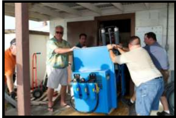
Bill Glynn, Charles Cable, James Polan, and Leonard Grandbois move the compressor onto a set of pipes so it can be slid through the door.
